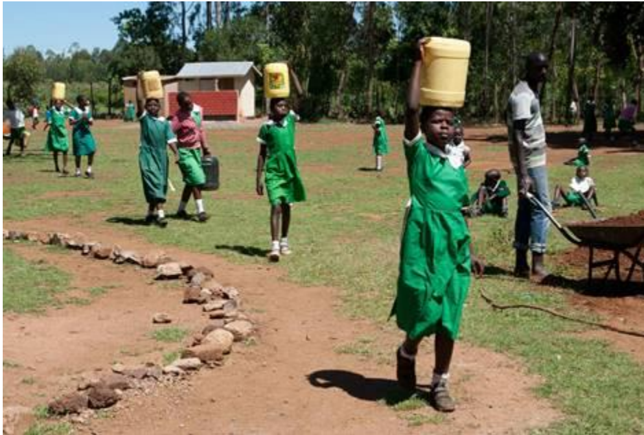
Some bigger girls were sent to a water source to haul water to the work site so that the cement could be mixed.
