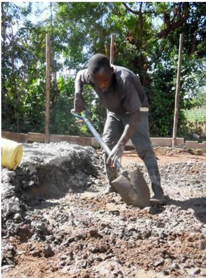
Any loose topsoil was scraped off, a course soil was added and pounded down, then the local laborers hand mixed the cement with a single shovel for the floors. This guy is wearing rubber boots but some of the others chose to do it in bare feet.
