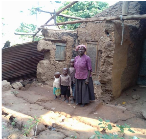
Ms. Aidah standing on her collapsed house
